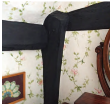
Beams in Sprimont House which would have supported the roof to the original cottage [Alan Brookes]
